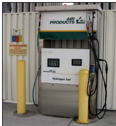
Figure 22. Compressed Hydrogen Dispenser
