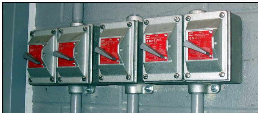
Figure 28. Explosion Proof Switches
