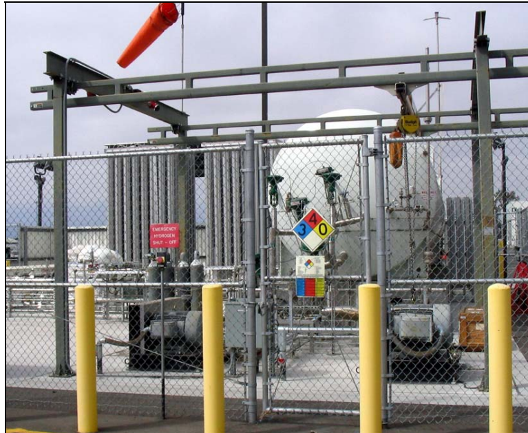
Figure 20. Liquid Hydrogen Storage Tank and Vaporizer
